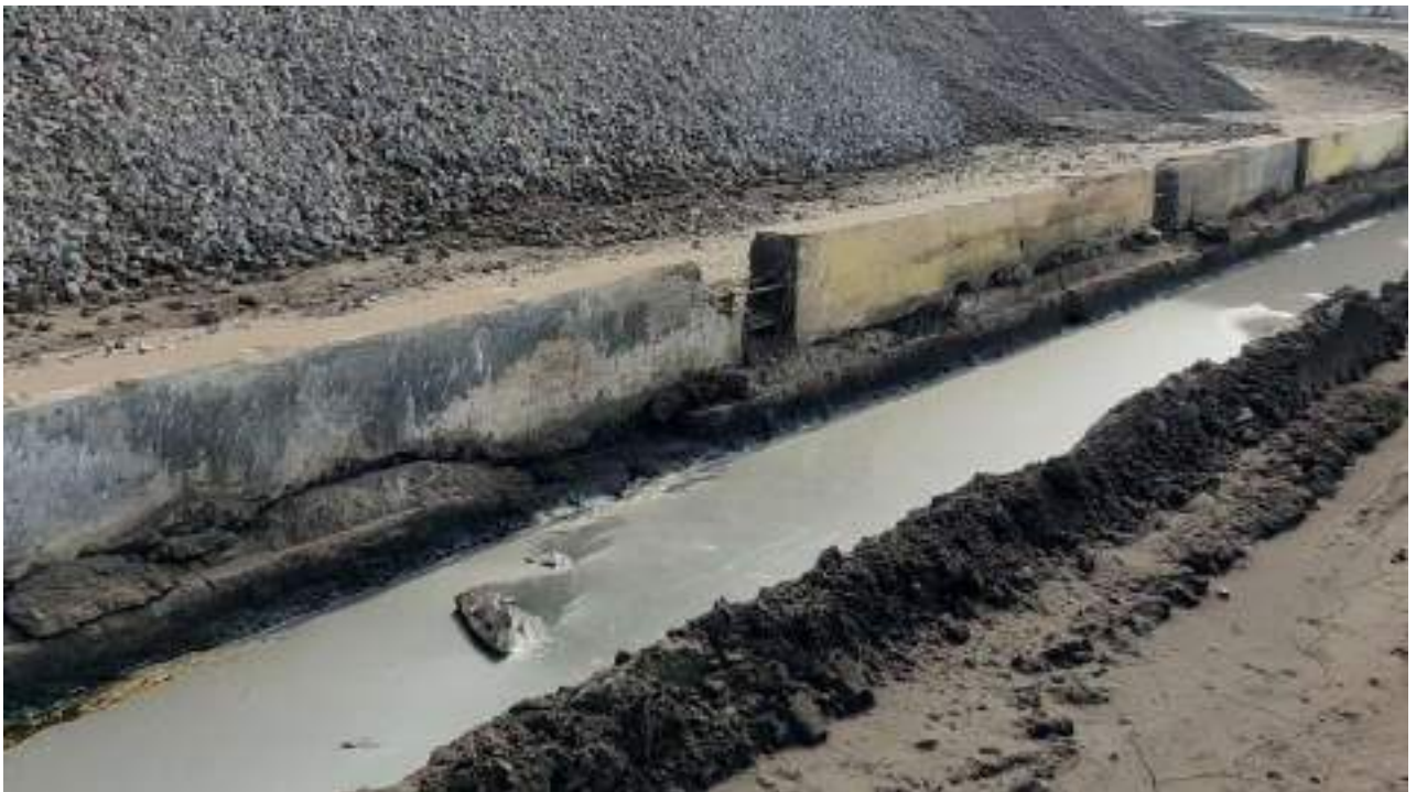
Fig. 7.7: Clogged storm water drain along coal yards
