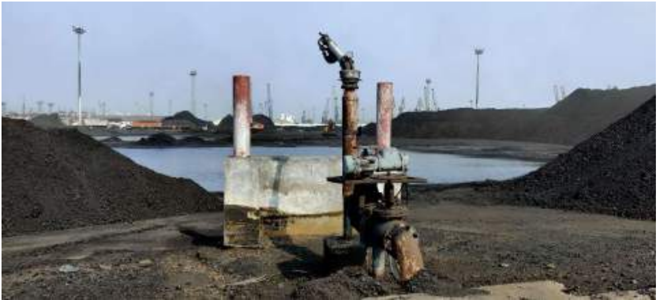
Fig. 7.6: Water sprinkler for suppression of coal dust
